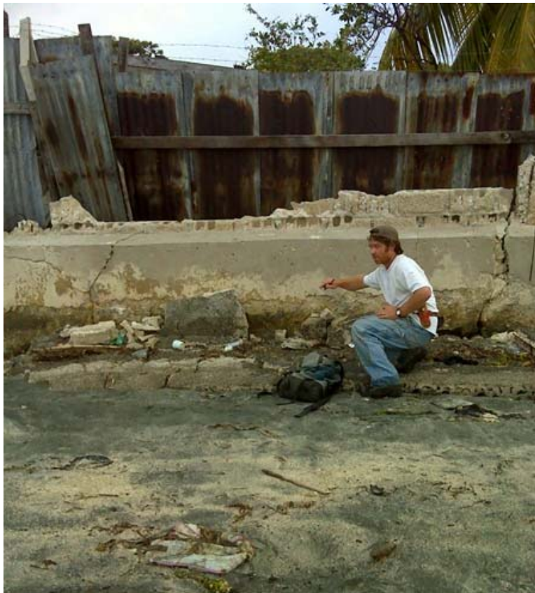
Figure 4.16. Water mark for high tides on sea wall at Ca Ira, Léogâne. Residents indicate high tides no longer extend up the wall to the former high tide level (N18.524924, W72.650871)
